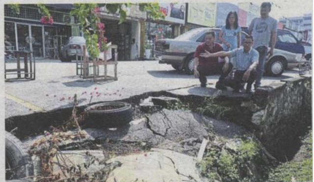
Yee showing part of the collapsed drain along Jalan Emas SD5/1B in Bandar Sri Damansara as affected business owners look on.
